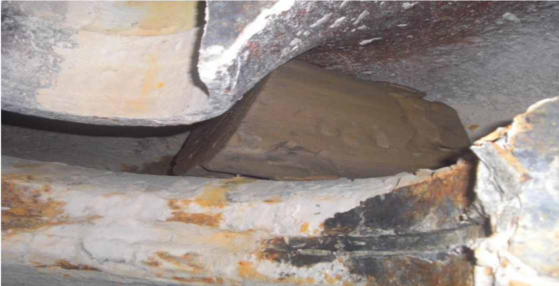
Figure 1. Pump casing status locked
