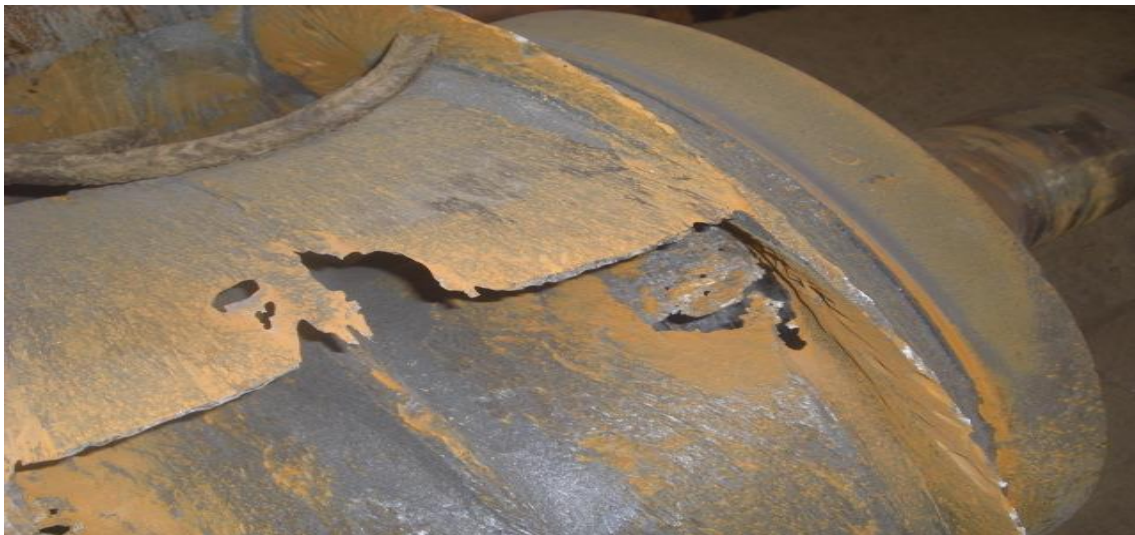
Rice. 2. Damage to the pump impeller due to cavitation erosion and hydroabrasive spreading 1-pump ishchi parragi; 2-cavitation eyelash
